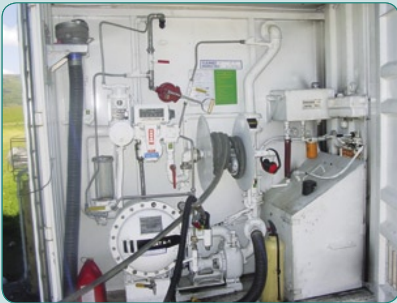
The high-flow fuel pump system used to refuel the incident aircraft. This system is capable of delivering fuel at a significantly higher rate than the standard fuel pumps found at most aerodromes.
