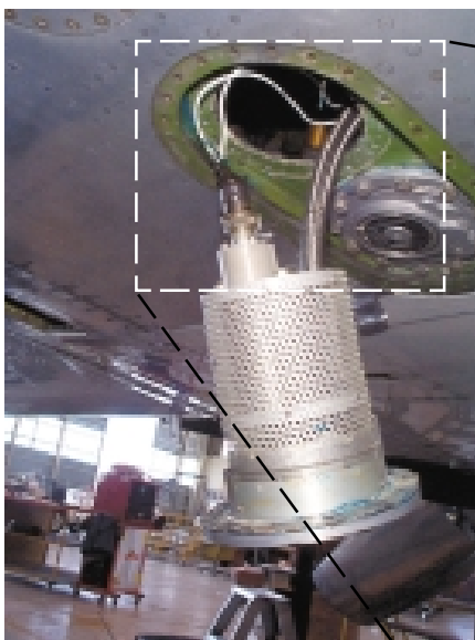
Chafed fuel booster pump wiring found inside the fuel tank of a Fairchild Metroliner following an emergency AD inspection.
